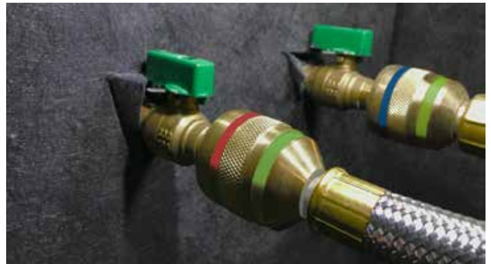
Colored ID bands to indicate supply and return water usage.
